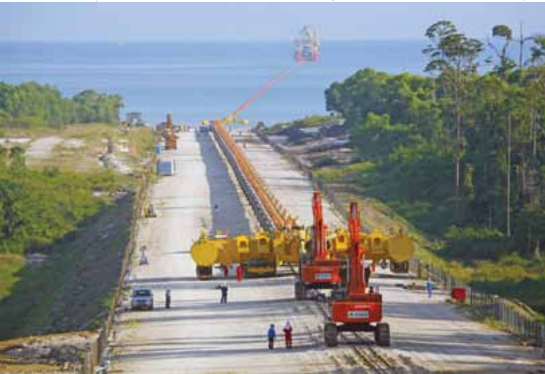
Kikeh Gap System Fabrication and Assembly of Gravity Actuated Pipeline System 2000 tonnes
