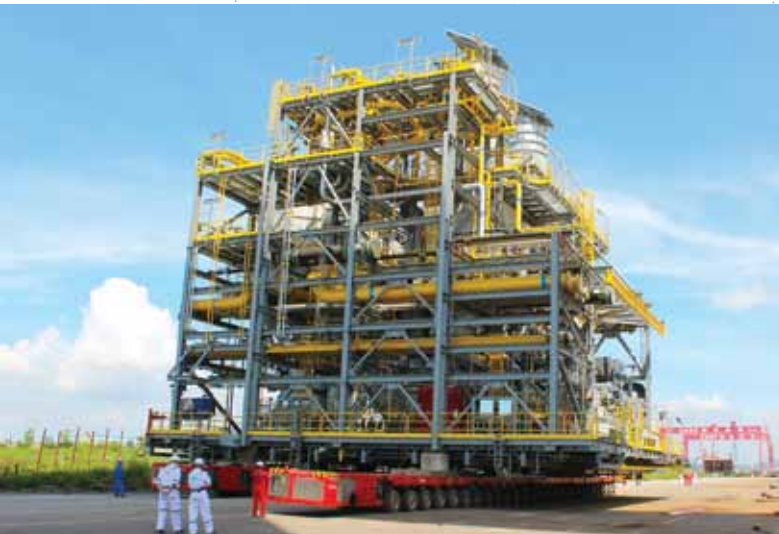
FPSO Cidade De Marica TS012 Power Generation B Module loaded out from yard
