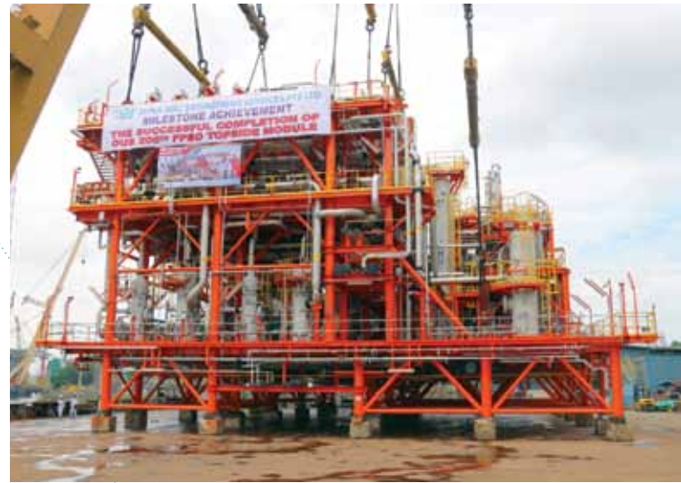
A key milestone with the load-out of the 200th Module in August 2014
