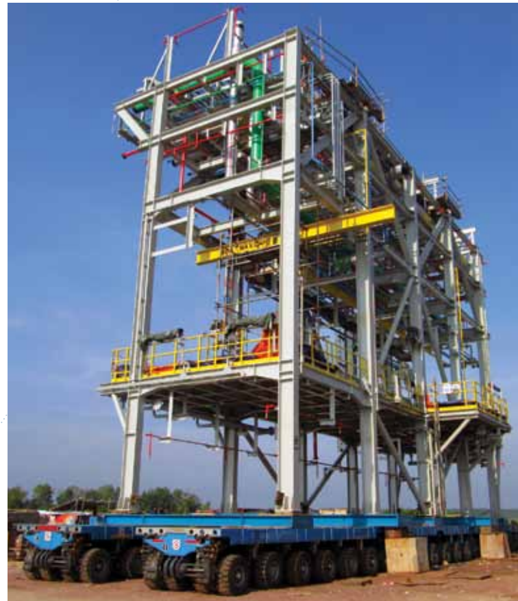
Ten Tullow Pipe Racks
