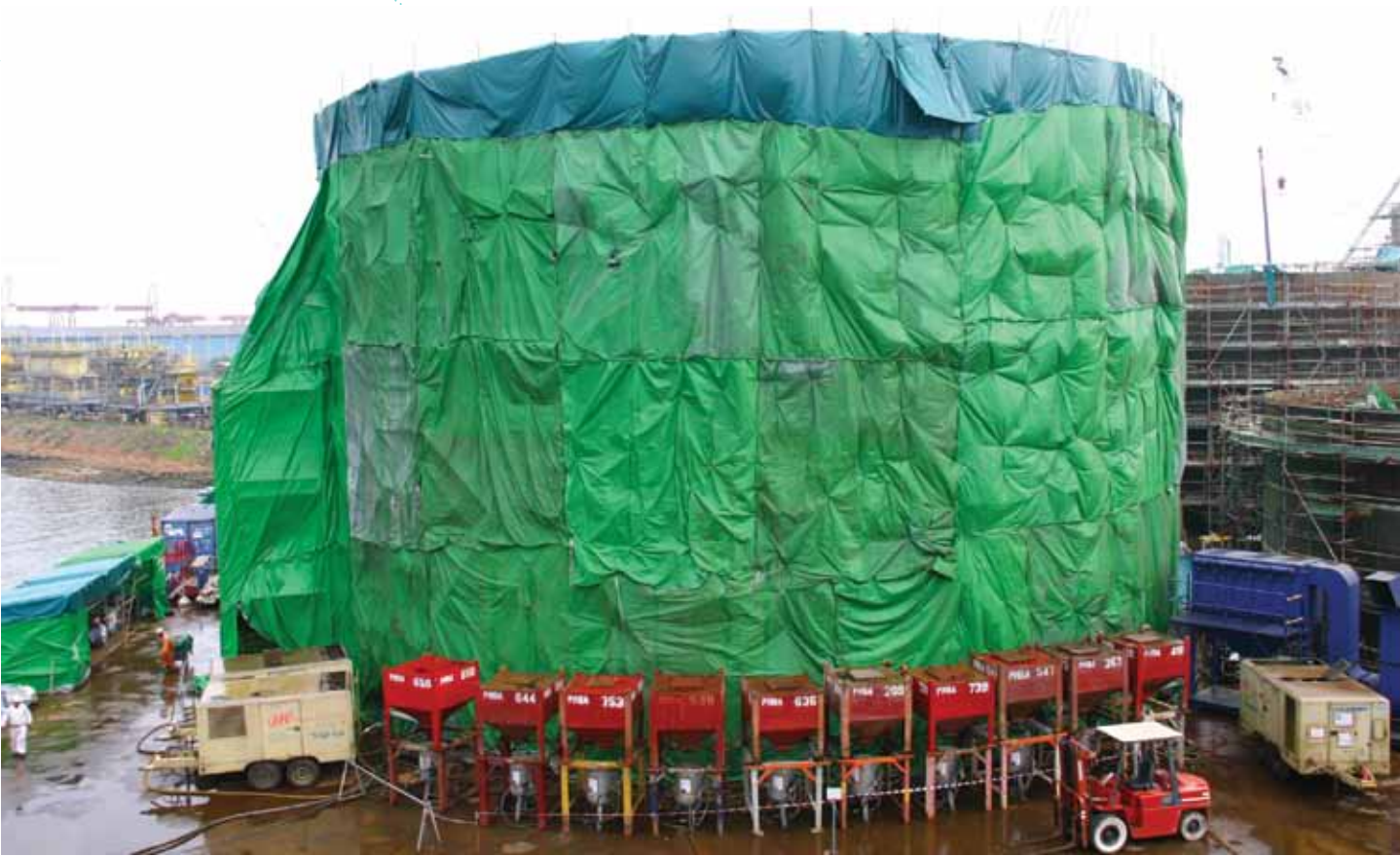
Effective dust containment and collection
