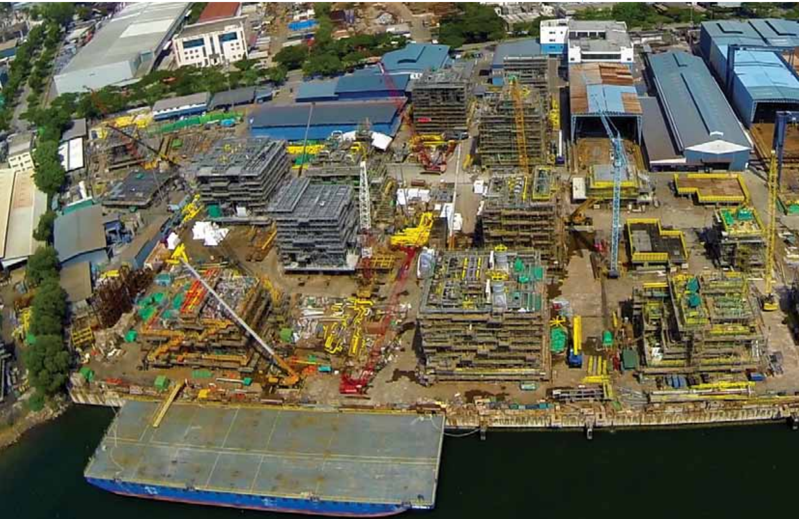
The Main Yard was kept busy with record deliveries of topside modules
